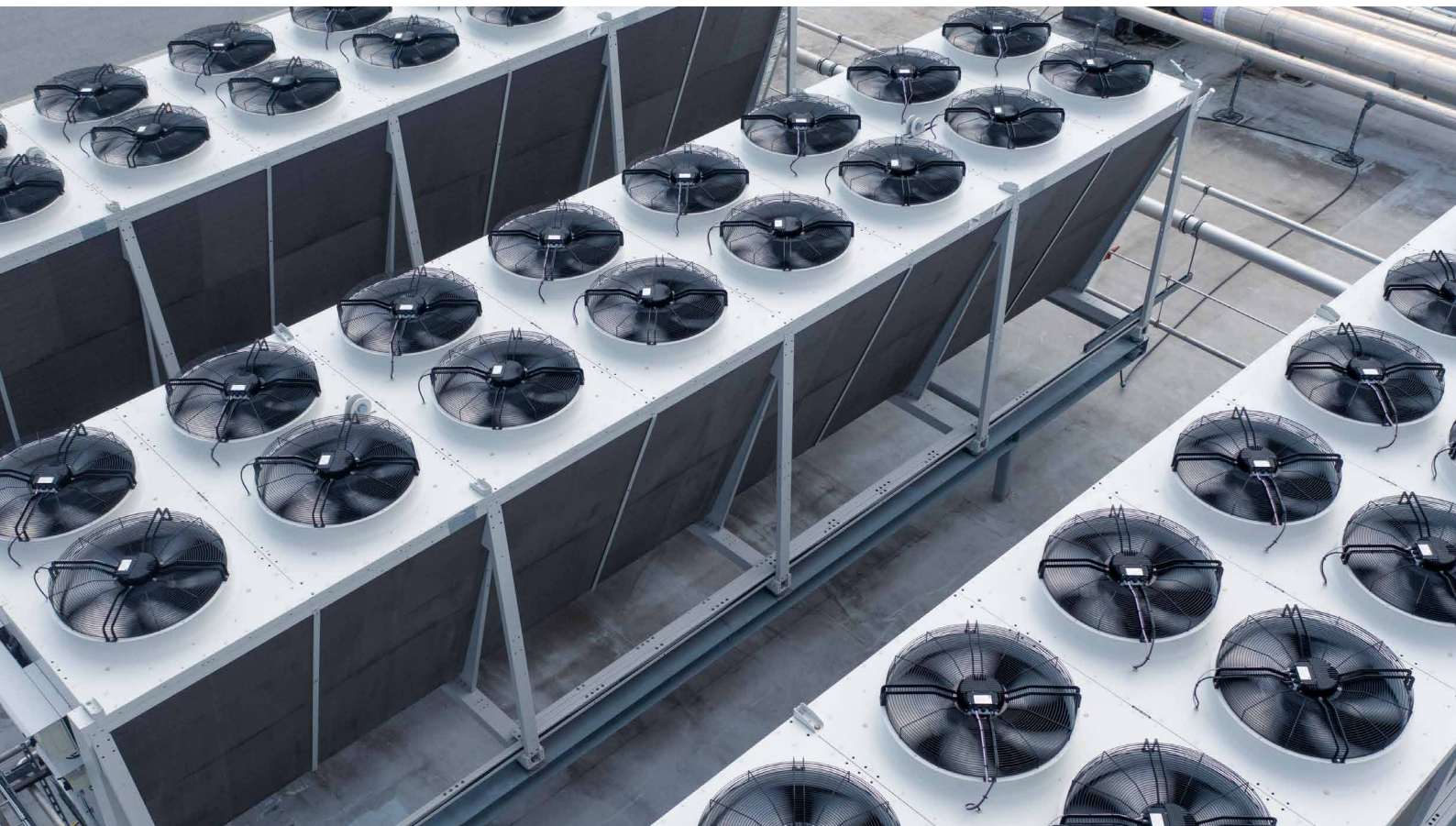
Cooling system of a large warehouse on the roof
